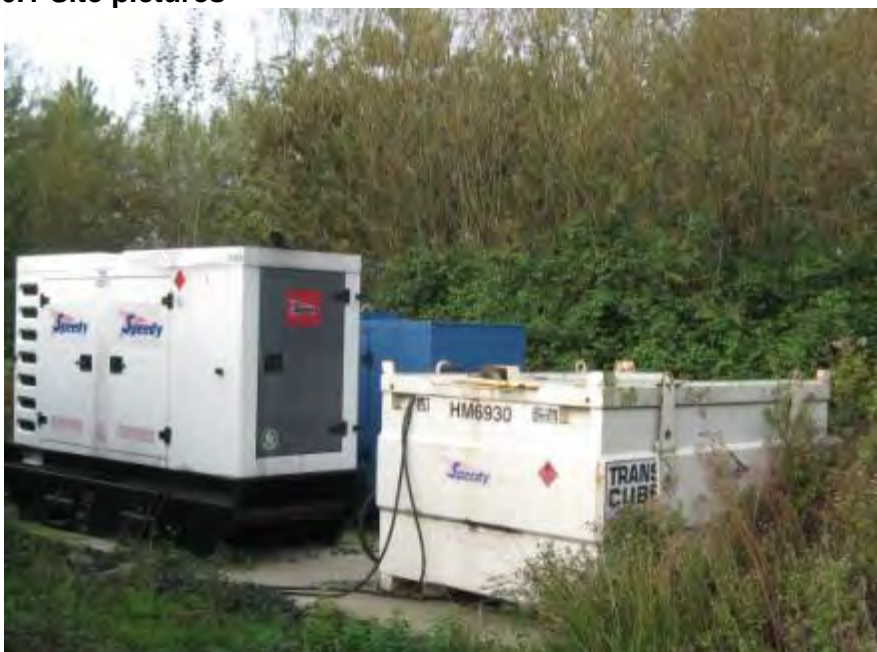
1. Site Generator package
