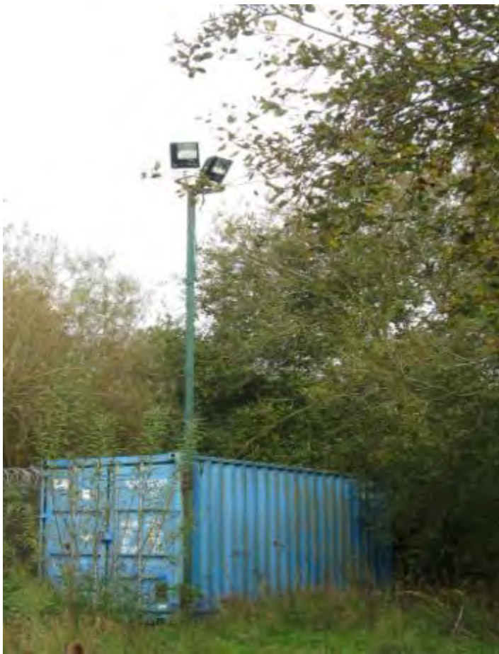
3 Site Lighting and electrical cabinet
