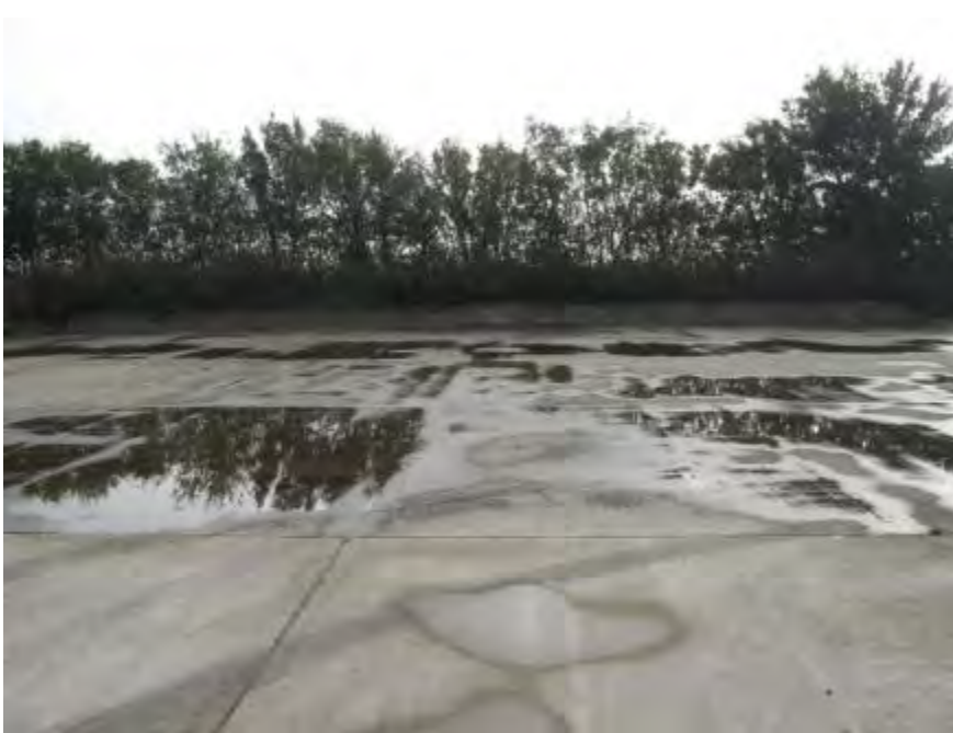
10, 11 Site lay down area to hold casing, seen below, temporarily awaiting drill of Lidsey 2.
