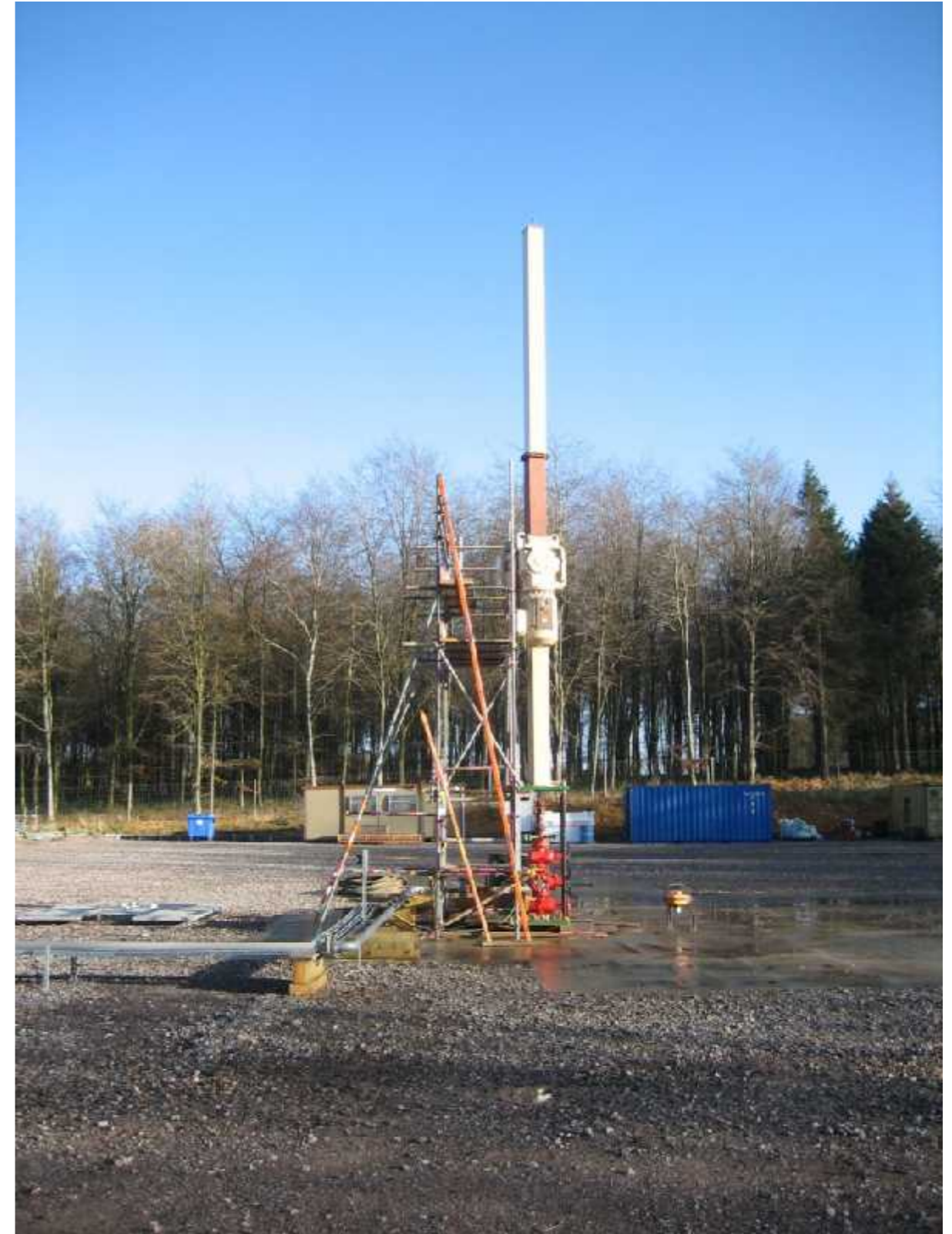
▲ Pumping unit installed on well for EWT with office and storage container in the background
