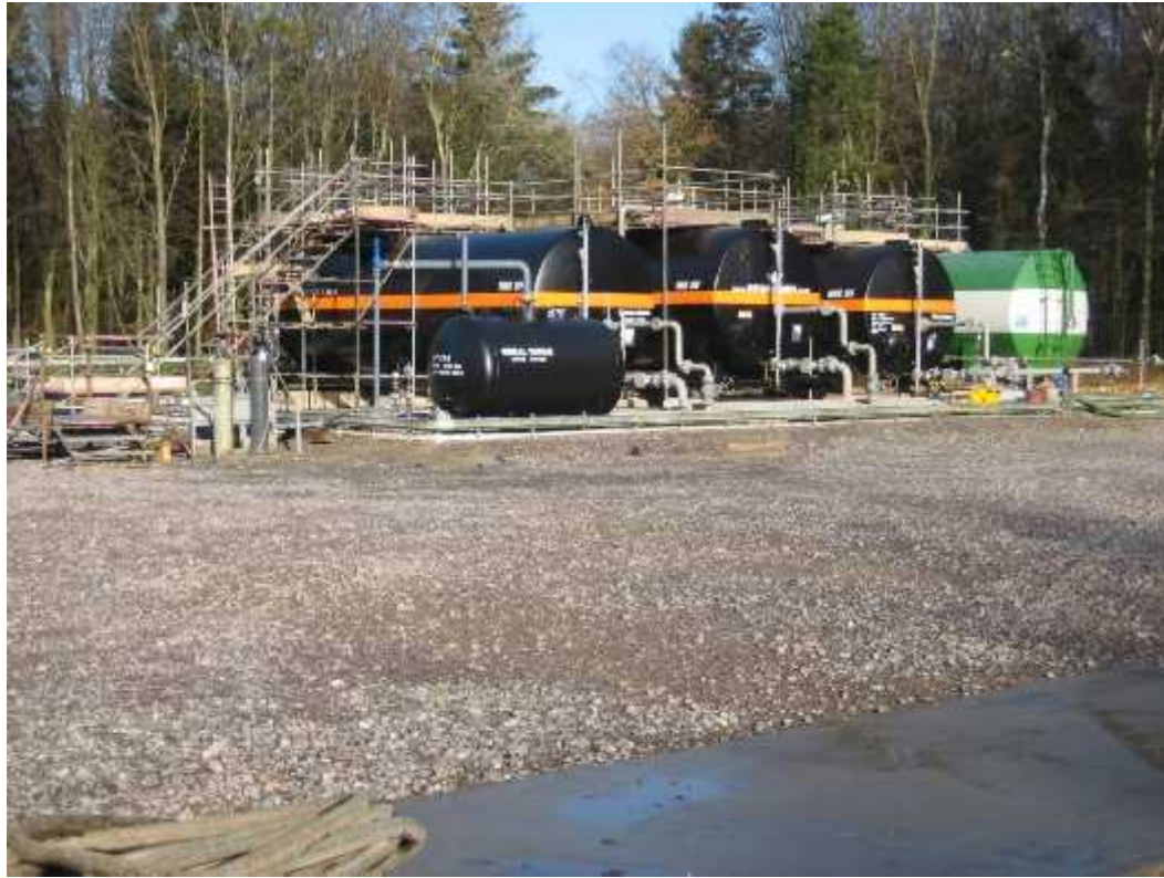
◀ Temporary Produced Oil and Water Storage tanks in a bunded area for an EWT with scaffolding access to permit tank sampling and measurements
