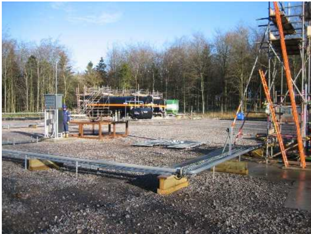
◀ General layout on the wellsite for EWT showing base of pumping unit on the right, pump control unit on the left and tanks in the background
