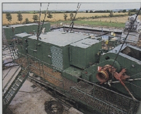
RIG ENGINE ACOUSTIC ENCLOSURE
