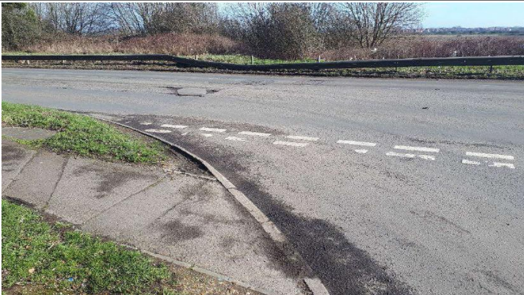
Photo J Ford Road carriageway markings illegible
