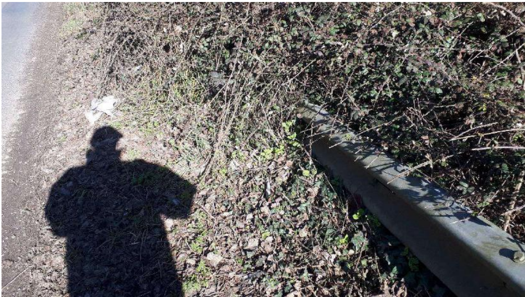
Photo B Existing damaged VRS non-compliant on east side of Ford Road
