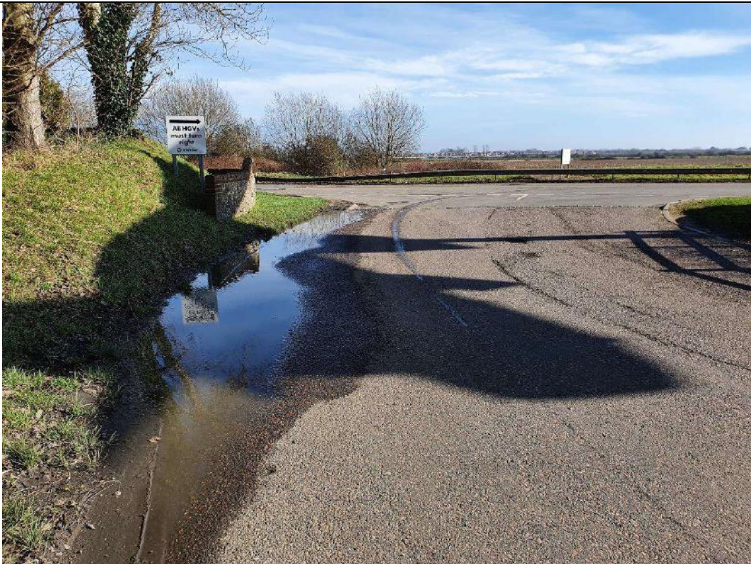
Photo D Ponding of water on site access road
