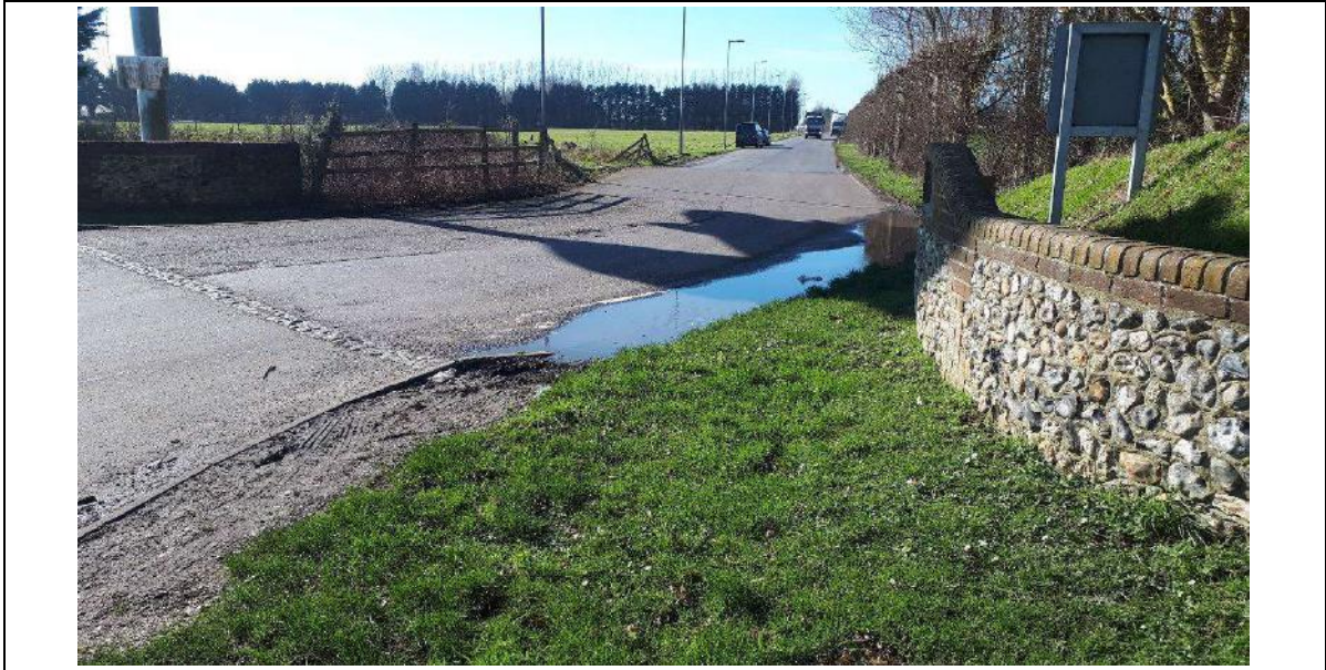
Photo E Ponding of water on site access road
