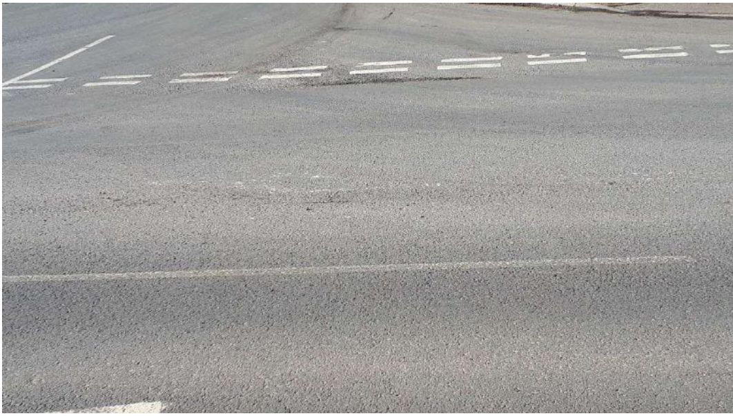
Photo M Ford Road carriageway markings illegible
