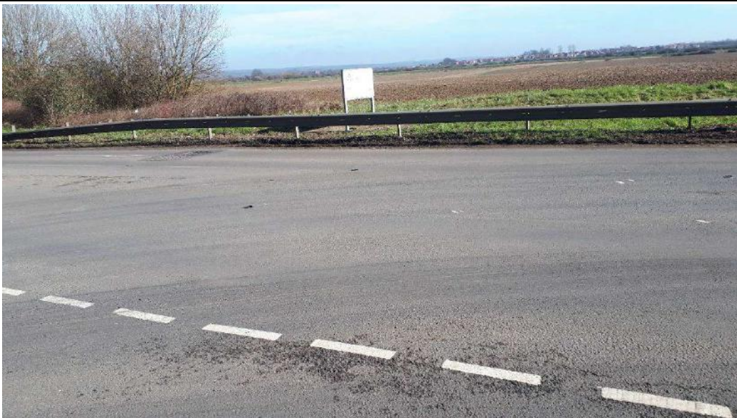
Photo L Ford Road carriageway markings illegible
