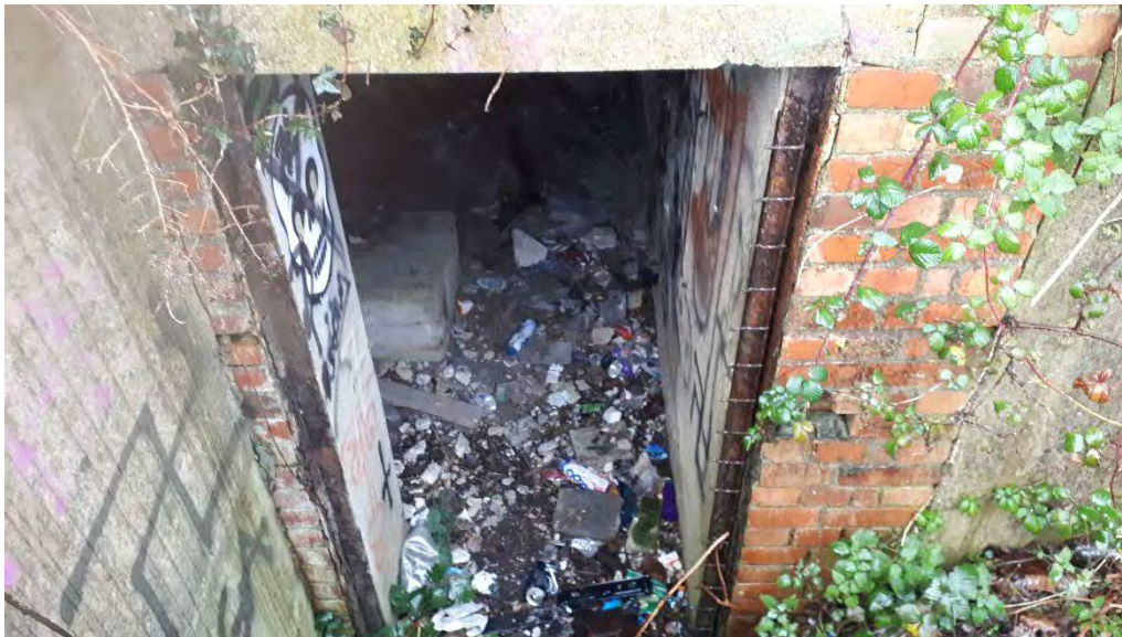
Photo 24. RAF Pumping Station/Bunker Filled with Fly Tipped Waste
