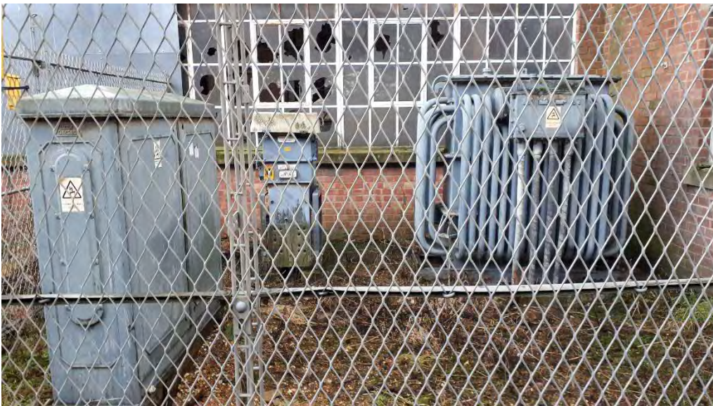
Photo 22. Electricity Sub-station (Hangar 2)
