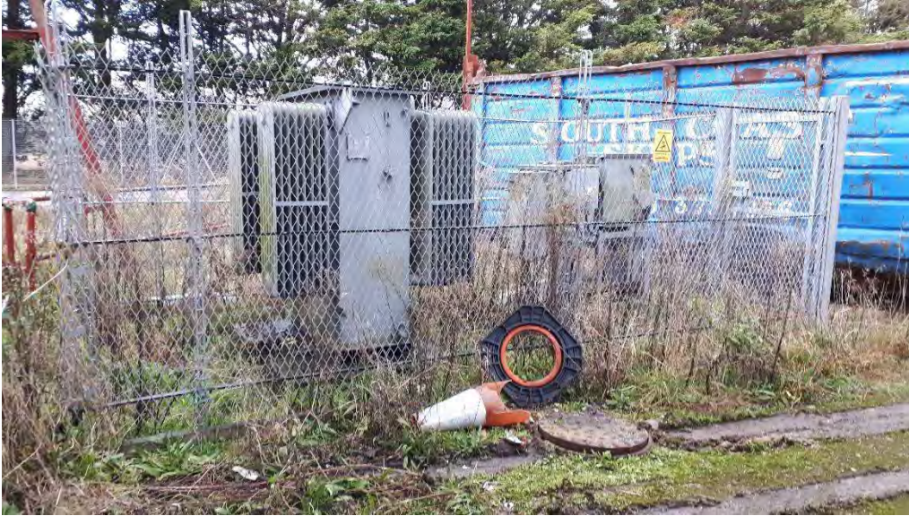
Photo 21. Electricity Sub-station (Hangar 1)
