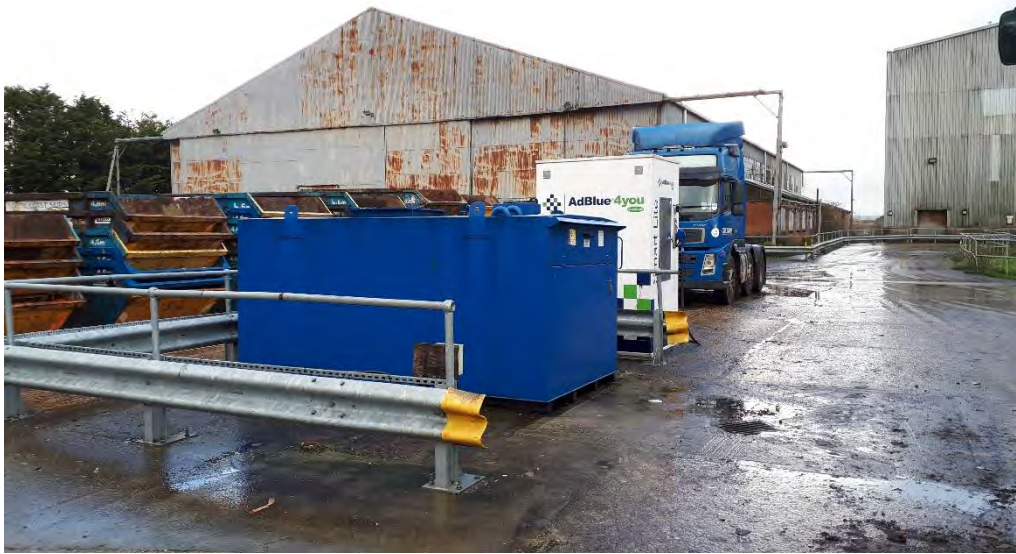
Photo 15. 5,600I Oil Tank
