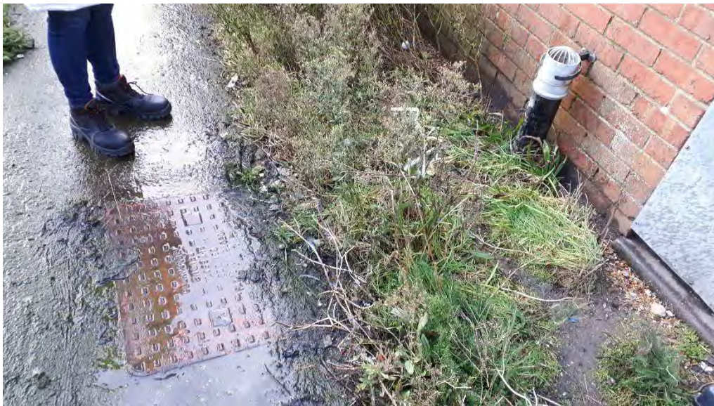
Photo 14. Cover Possibly Indicating the Presence of an Interceptor or Underground Storage Tank Adjacent to Hangar 2
