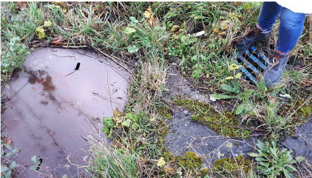
Photo 12. Cover Possibly Indicating the Presence of an Interceptor or Underground Storage Tank Adjacent to Hangar 2
