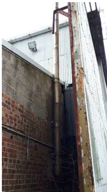
Photo 20. Disused Metal Piped Chimney
