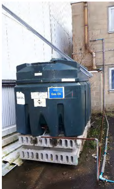
Photo 16. 2,500I Gas Oil Tank
