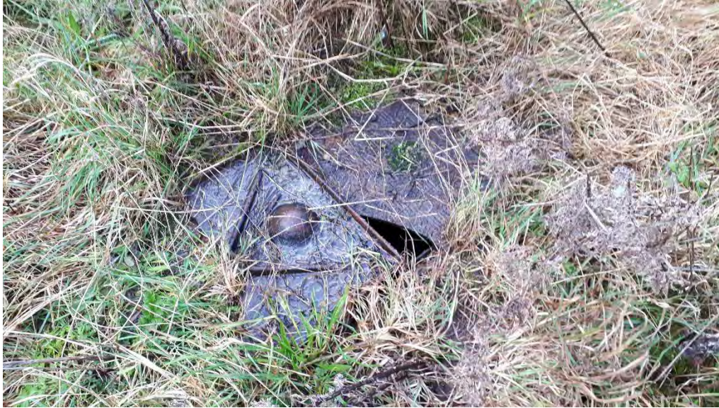
Photo 13. Cover Possibly Indicating the Presence of an Interceptor or Underground Storage Tank Adjacent to Hangar 2
