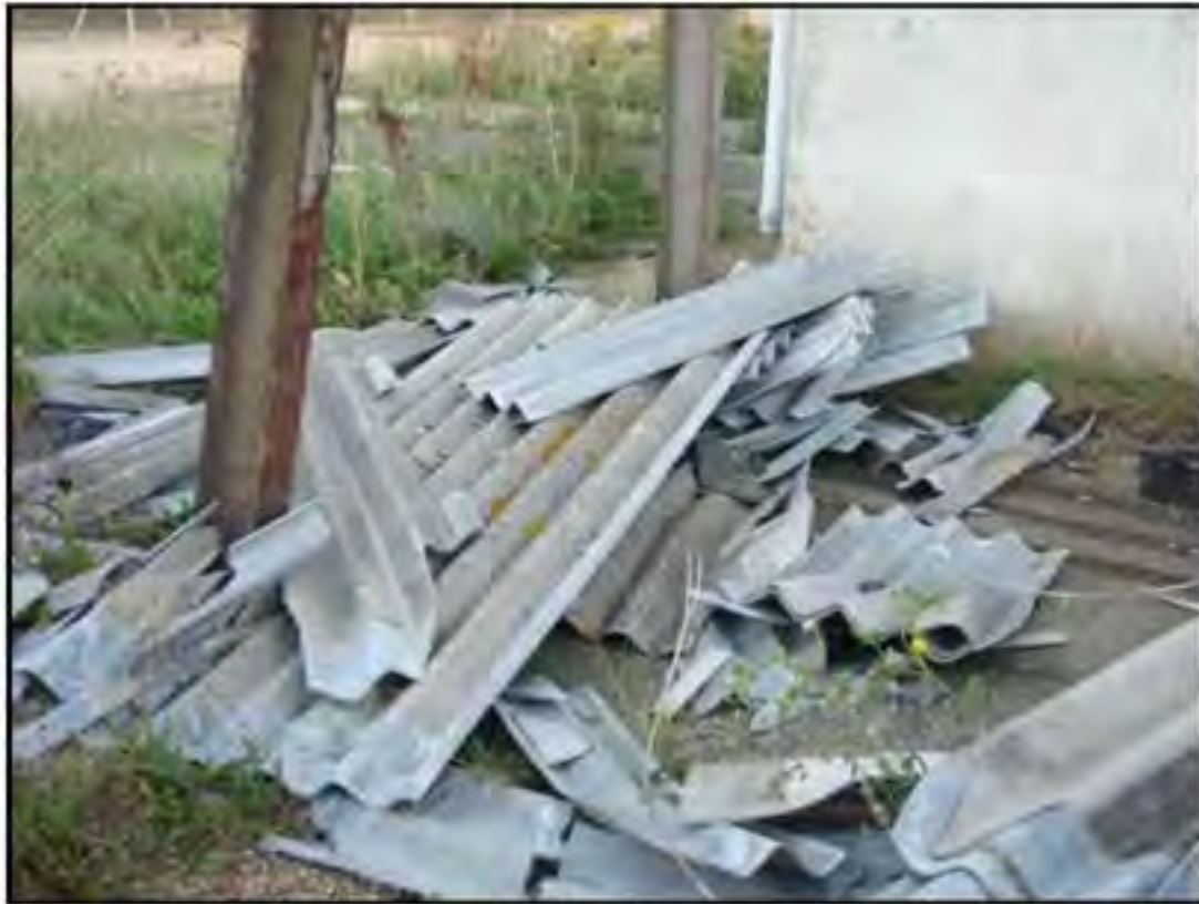
Plate 17: Asbestos sheeting adjacent to North West corner - Hangar 1.
