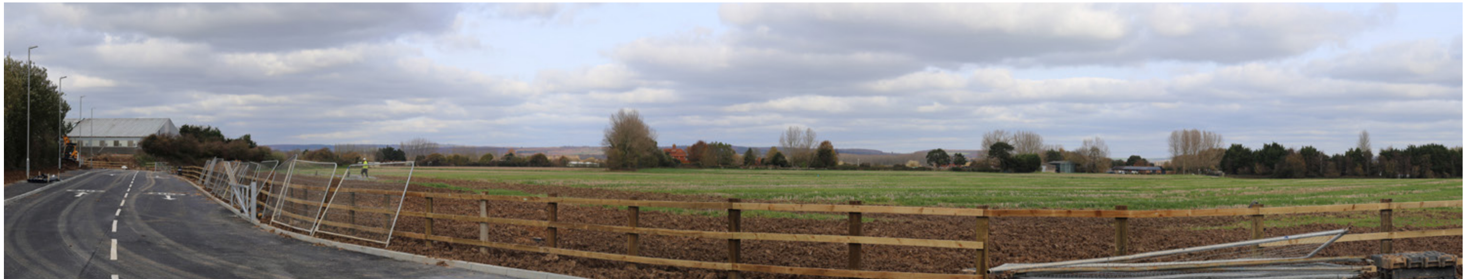
The new access road under construction, and view towards the rear of the buildings along Ford Lane
