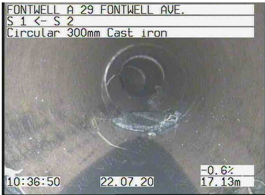
S 1X_5ea0d0dc-ae2d-4172-9971-a51fbc440884_20200722_103841_992.jpg, 00:01:13, 17.13 m Roots, fine at joint
