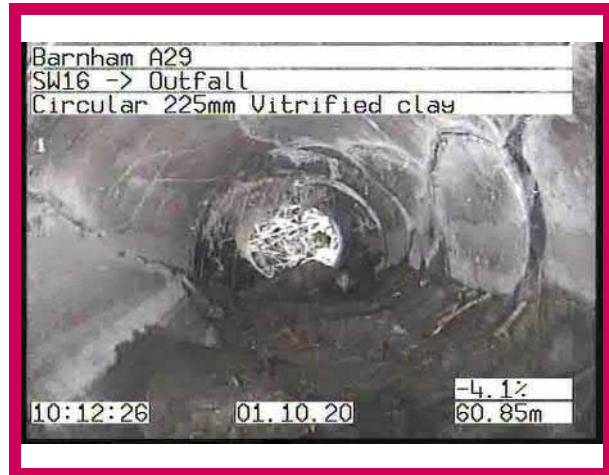
4, 00:08:34, 60.84 m Fracture, multiple from 8 o'clock to 4 o'clock
