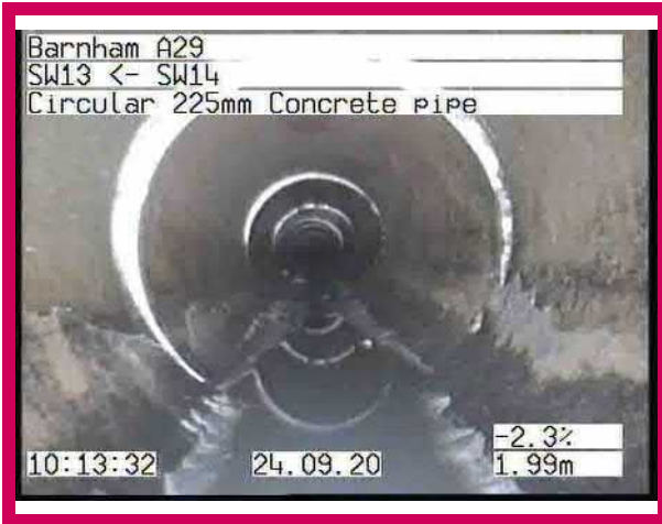
1, 00:00:26, 2.17 m Joint displaced, medium
