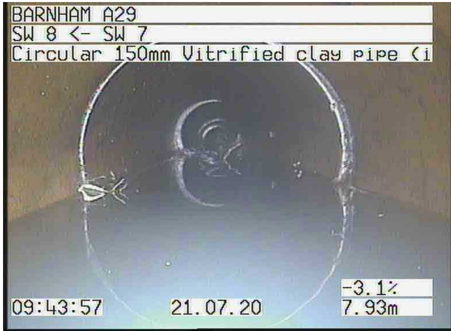
SW 8X_8c4988ac-d5d1-485b-bb90-dfc661fdb8d7_20200721_094546_267.jpg, 00:01:30, 7.52 m Connection other than junction at 12 o'clock, diameter: 150mm
