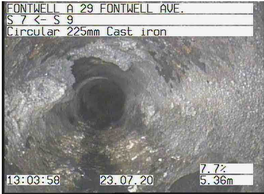
S 7X_35ac63c3-dec3-455f-8215-92d252d94c64_20200723_130537_508.jpg, 00:00:28, 5.36 m Attached deposits, encrustation from 9 o'clock to 10 o'clock, 20% cross-sectional area loss
