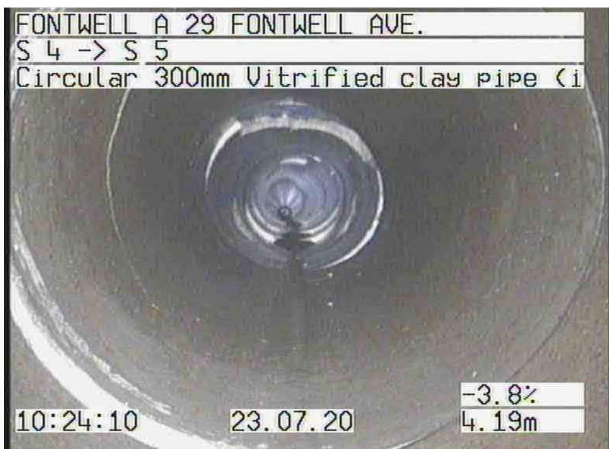
S 4X_e8687c64-3f97-495e-9180-552d6f4f3cce_20200723_102549_074.jpg, 00:00:36, 4.19 m Fracture, circumferential from 7 o'clock to 12 o'clock
