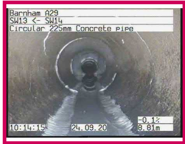
2, 00:00:57, 8.81 m Fracture, circumferential from 9 o'clock to 5 o'clock
