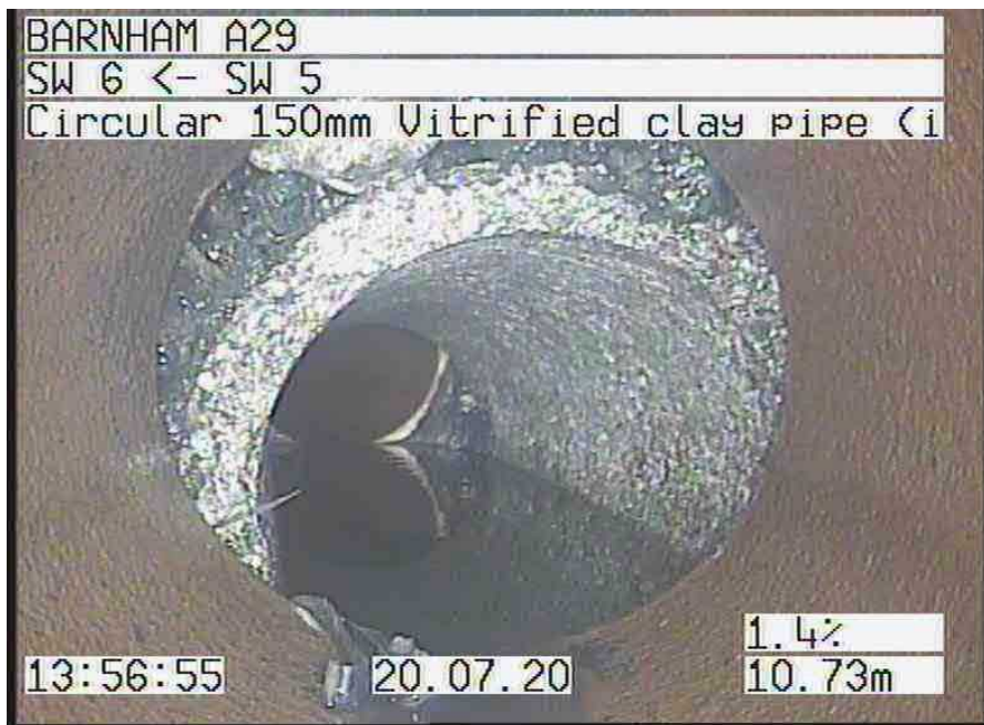
SW 6X_bd285a99-d44c-41d8-b85f-d6ec17a81367_20200720_135842_190.jpg, 00:01:16, 10.73 m Survey abandoned, DUE TO DISPLACED JOINT
