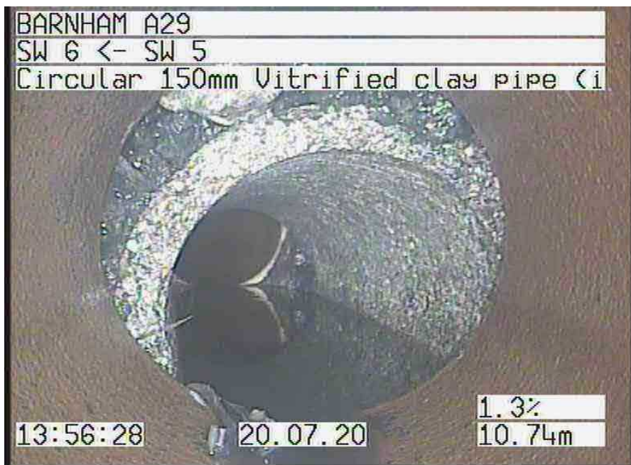
SW 6X_40db77c5-630e-4145-a098-f774cc199496_20200720_135815_263.jpg, 00:01:11, 10.76 m Joint displaced, large
