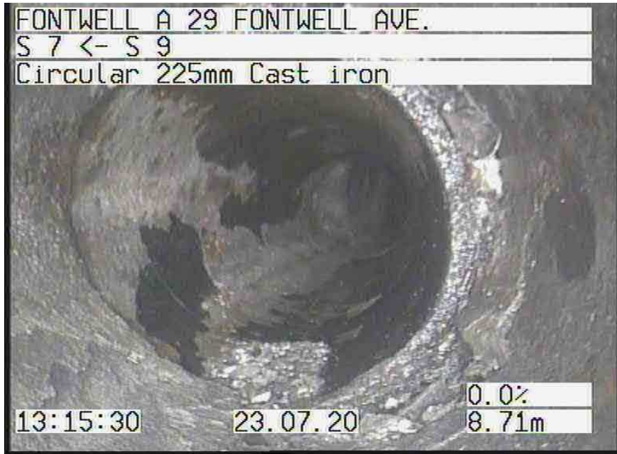
S 7X_1d069ccc-2753-4800-850e-0dc77471c39a_20200723_131709_472.jpg, 00:00:46, 8.71 m
