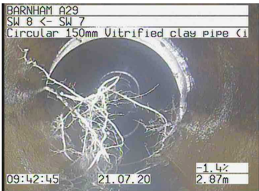
SW 8X_2c402511-4646-4751-b995-ba44b1e1f689_20200721_094434_200.jpg, 00:00:50, 2.87 m Roots, tap at joint
