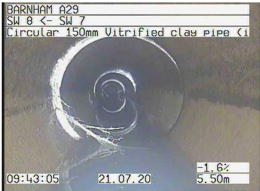
SW 8X_1be65c57-f970-4dd4-a9bd-98954347378e_20200721_094454_109.jpg, 00:01:08, 5.44 m Roots, tap at joint
