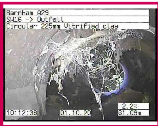
5, 00:08:45, 61.09 m Broken pipe from 10 o'clock to 2 o'clock
