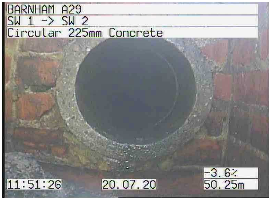
SW 1X_5e075df2-8536-40dc-8176-e38cc8cc59e1_20200720_115312_964.jpg, 00:04:08, 50.25 m Finish node type, catchpit, reference number: SW 2
