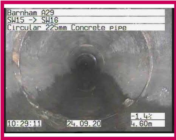
1, 00:00:28, 4.59 m Fracture, longitudinal at joint at 12 o'clock
