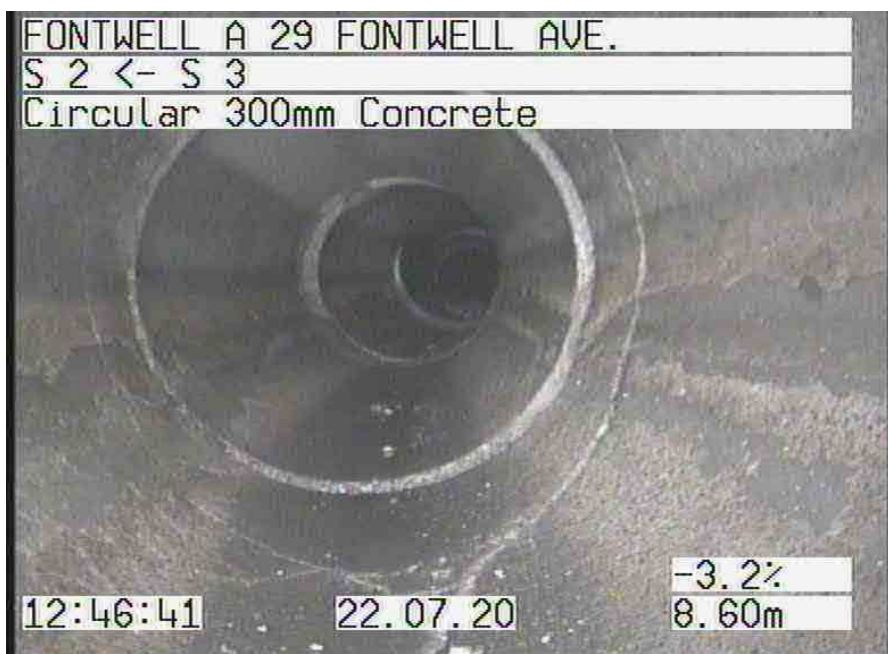
S 2X_f77ccb20-a914-4af1-ab59-3e44fb45e56f_20200722_124833_240.jpg, 00:01:17, 8.60 m Fracture, circumferential from 12 o'clock to 12 o'clock
