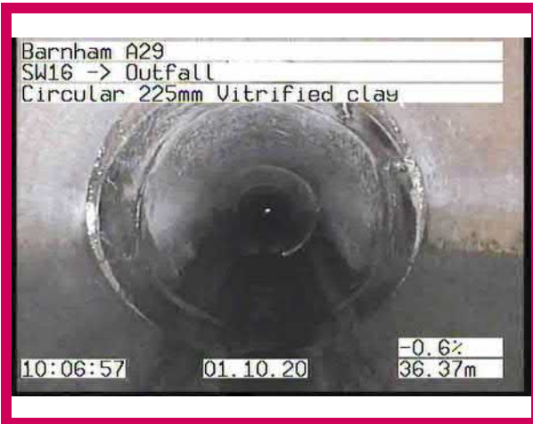
3, 00:03:48, 36.73 m Fracture, circumferential at joint from 8 o'clock to 3 o'clock
