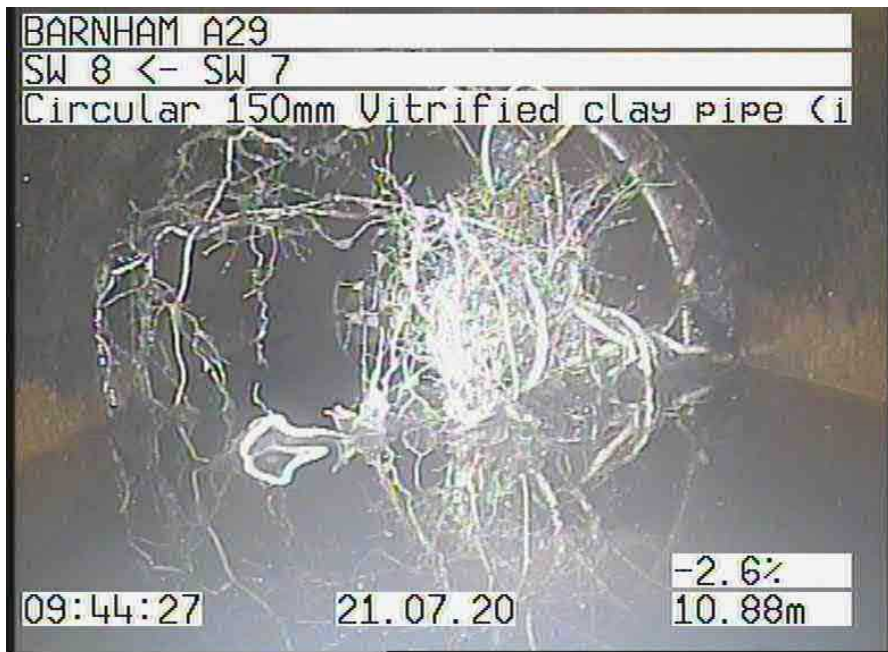
SW 8X_95cd1bcc-af66-4697-abb0-e04089c135fd_20200721_094616_416.jpg, 00:02:01, 10.88 m Roots, mass, 30% cross-sectional area loss
