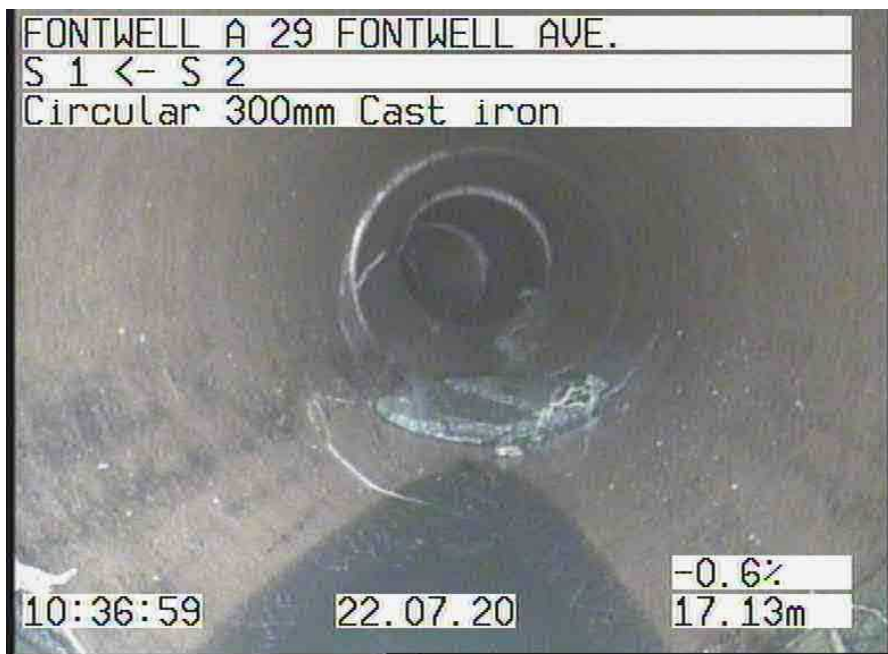
S 1X_9eb05902-a84d-450c-8bfe-67dbfd30245a_20200722_103850_088.jpg, 00:01:19, 17.13 m Material changes to vitrified clay
