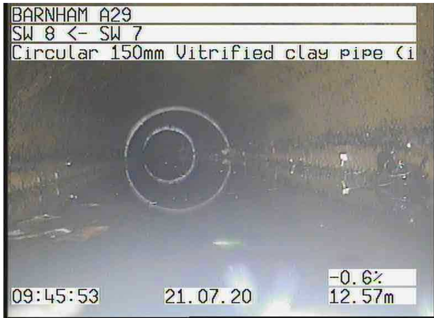
SW 8X_fb604b83-734b-4655-a3ef-4f075f8793a9_20200721_094742_587.jpg, 00:03:03, 12.57 m Survey abandoned, DUE TO ROOT MASS
