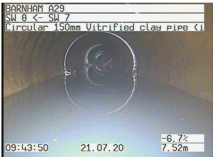
SW 8X_2aede51-6404-4cd3-bfcf-a823d2e5c3b5_20200721_094539_394.jpg, 00:01:24, 7.20 m Water level, 30% of the vertical dimension
