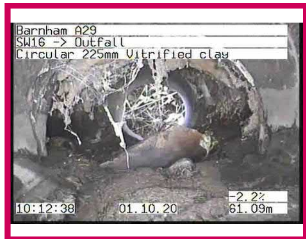
6, 00:08:45, 62.00 m Settled deposits, fine, 20% cross-sectional area loss
