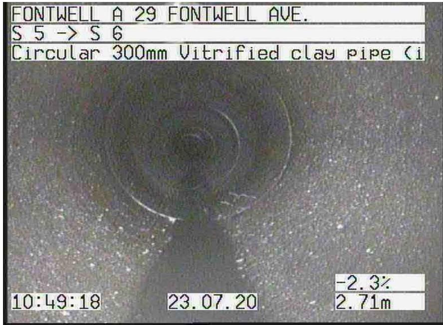
S 5X_a9b8138b-f5b7-4906-9384-e0eeeb86effb_20200723_105056_556.jpg, 00:00:23, 2.71 m
