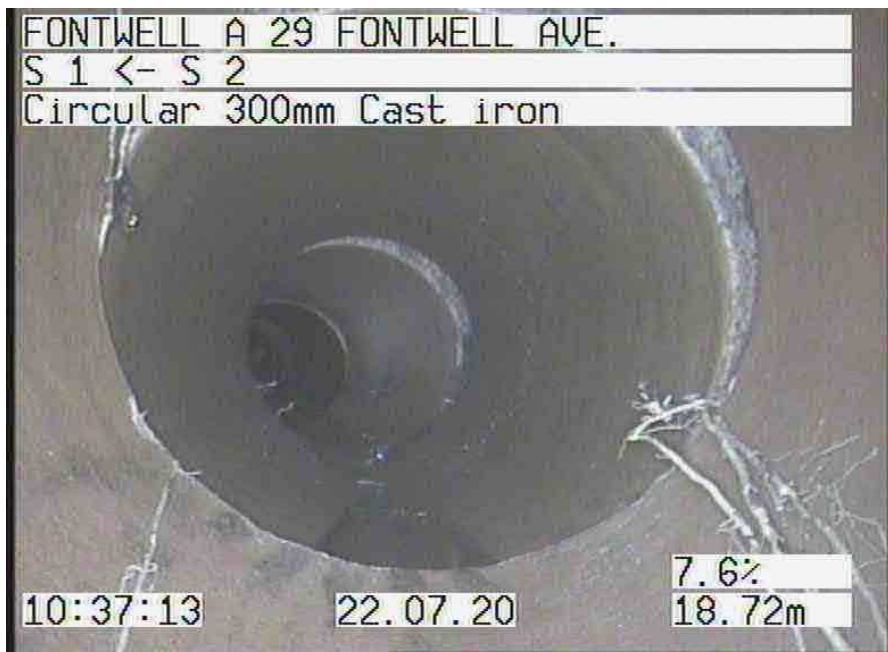
S 1X_1d6a4940-240e-46a7-848b-5f165be5c0d1_20200722_103904_219.jpg, 00:01:31, 18.72 m Roots, tap at joint
