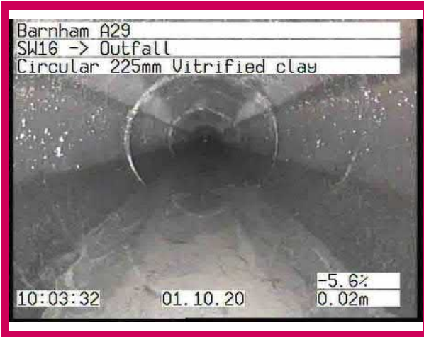
1, 00:00:22, 0.10 m Settled deposits, fine, 20% cross-sectional area loss, start
