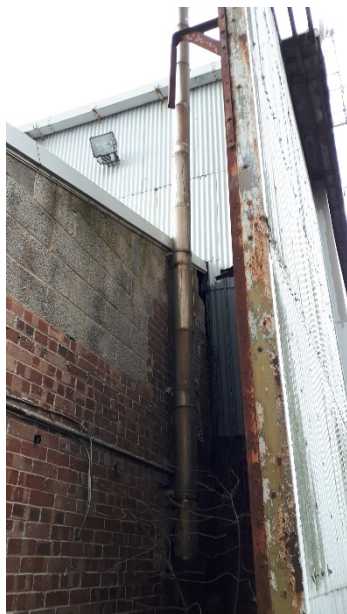
Photo 20. Disused Metal Piped Chimney
