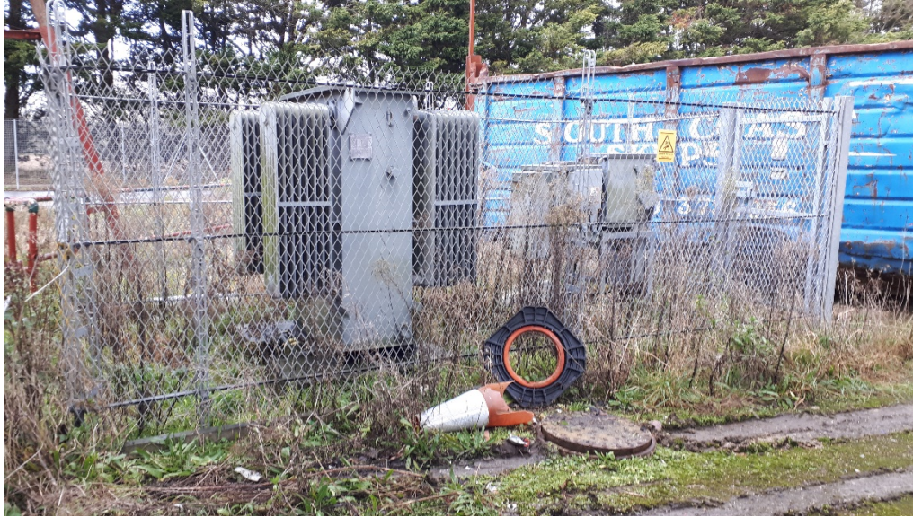
Photo 21. Electricity Sub-station (Hangar 1)
