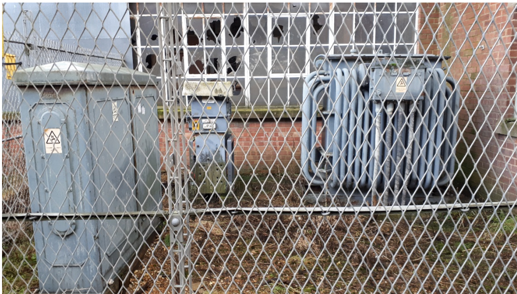
Photo 22. Electricity Sub-station (Hangar 2)
