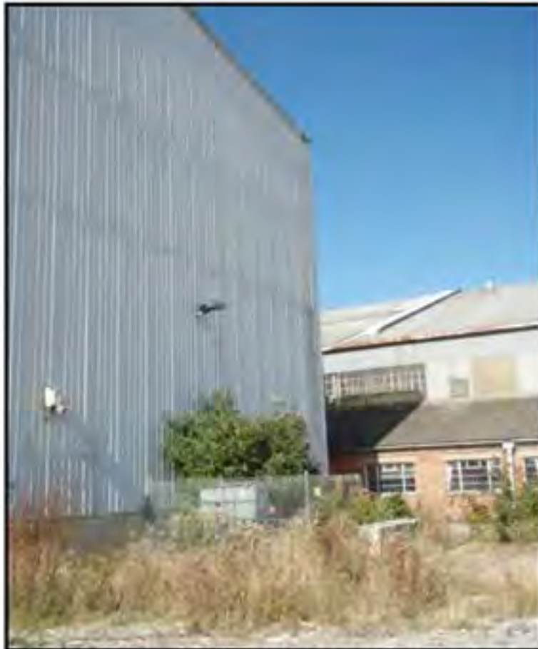
Plate 9: Sub Station adjacent to Aerated Block Plant - Hangar 3 and area of former slurry pit in the foreground.
