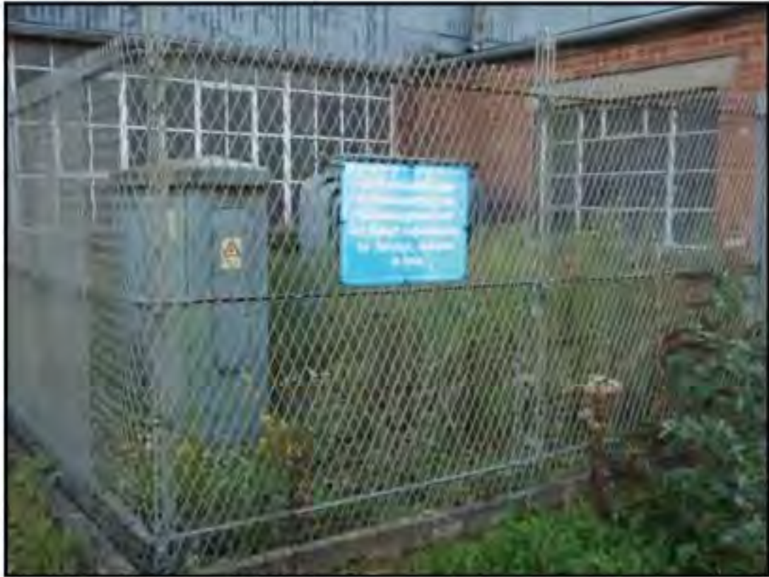
Plate 7: Sub Station adjacent to Hangar 2.
