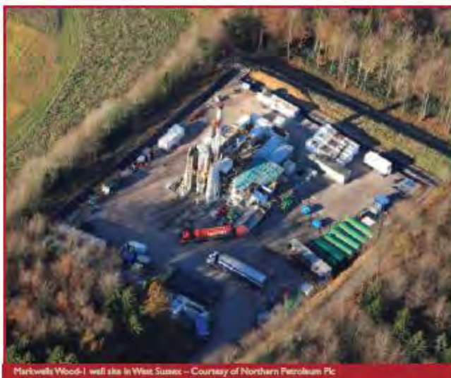
Markwells Wood-1 well site in West Sussex – Courtesy of Northern Petroleum Plc
