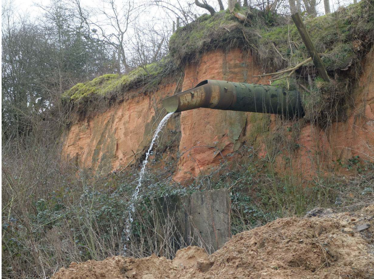
Figure A: Surface water entering site via drain on southern boundary
