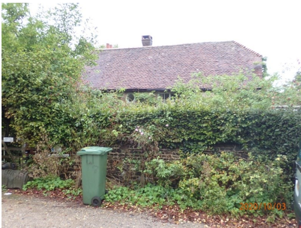
Plate 2: View of the Grade II listed Green Farmhouse, (Site No. 13), from the east
