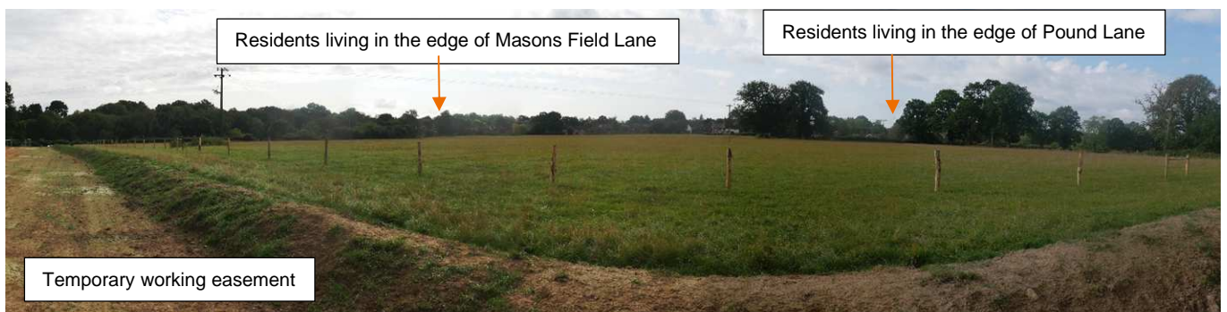
Photo 3: Taken from temporary construction road, looking south towards temporary working easement and residential properties.
