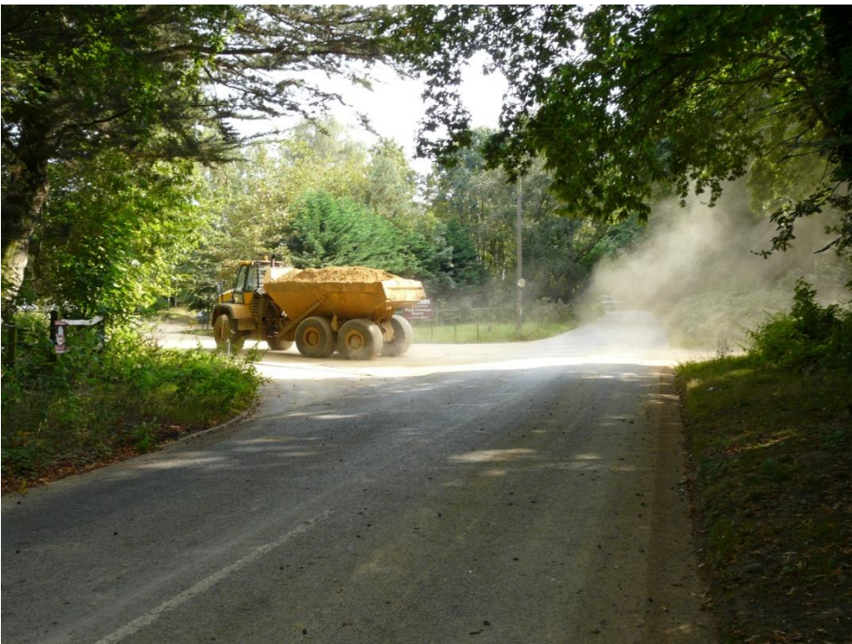
Road crossing not using conveyor belt contravening planning condition WS/15/97 #7 (2015)
