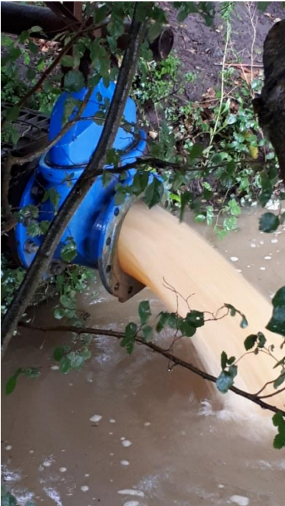
Silted water discharged to stream (October 2021)
