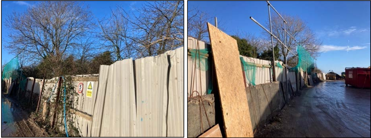
Photograph 8a (left) & b (right). The northern boundary of the existing recycling centre, showing the current corrugated metal, timber and chipboard fencing separating the site from the ditch.
